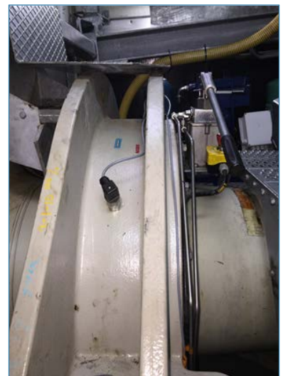
Figure 1. One of the accelerometers on the main bearing of a wind turbine at the Lone Star wind farm in Texas, USA.
