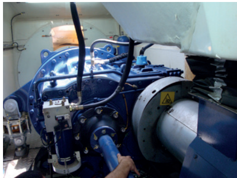
Figure 1. Site survey for installing the monitoring system hardware and sensors in the different types of wind turbines (left to right: Gamesa Type 1, Gamesa Type 2).
