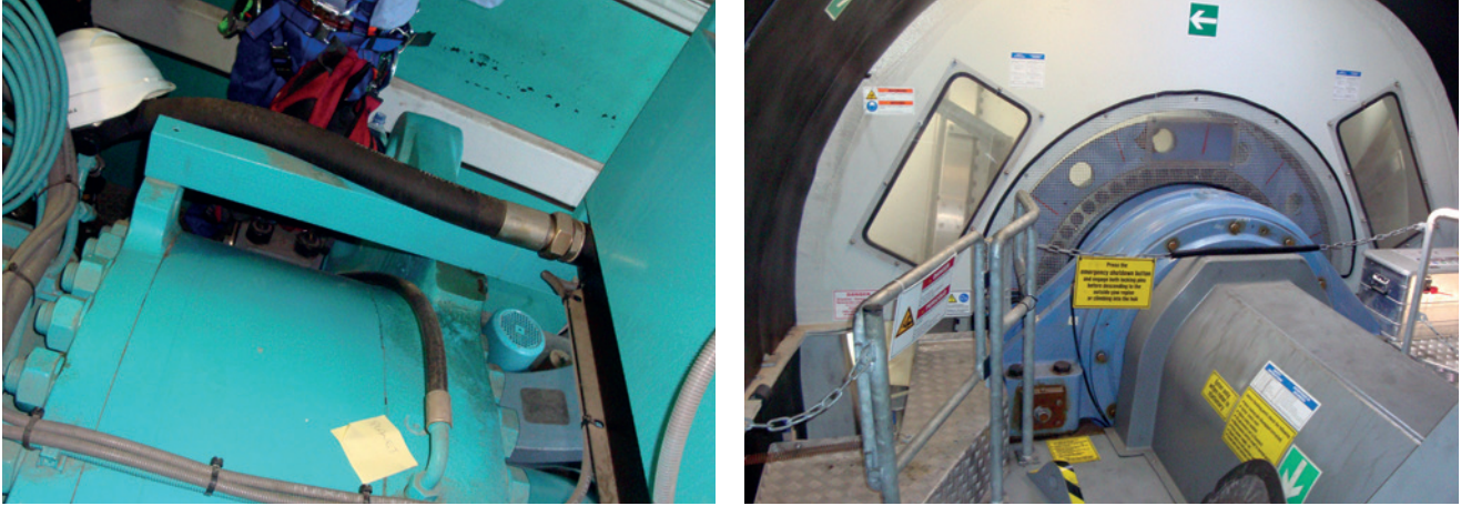
Figure 2. Site survey for installing the monitoring system hardware and sensors in the different types of wind turbines (left to right: GE 1.5 S, Repower).
