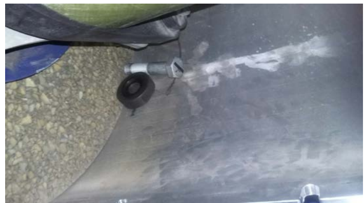
Figure 5: A coupling bracket bolt was found inside the coupling shield.
