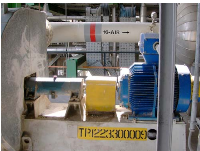
Fig. 1 Air compressor for the polyethylene line
