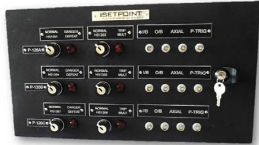
Figure 9: Door for 16-position rack with custom patch panel, trip multiply, and danger defeat switches/annunciators.
