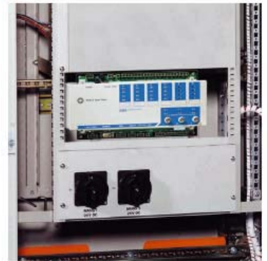
Figure 4. Cabinet installation in a safe area.
