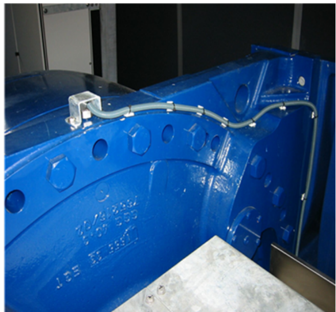
The required information and its use. To the right, an example of a sensor on a gearbox.
