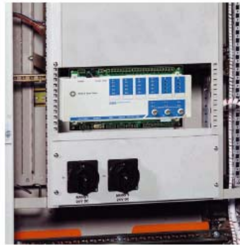
Fig. 4 Cabinet installation in a safe area
